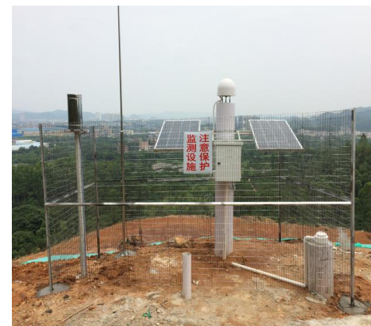
Displacement monitoring station and rainfall station
