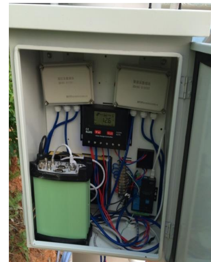
Internal picture of equipment cabinet
