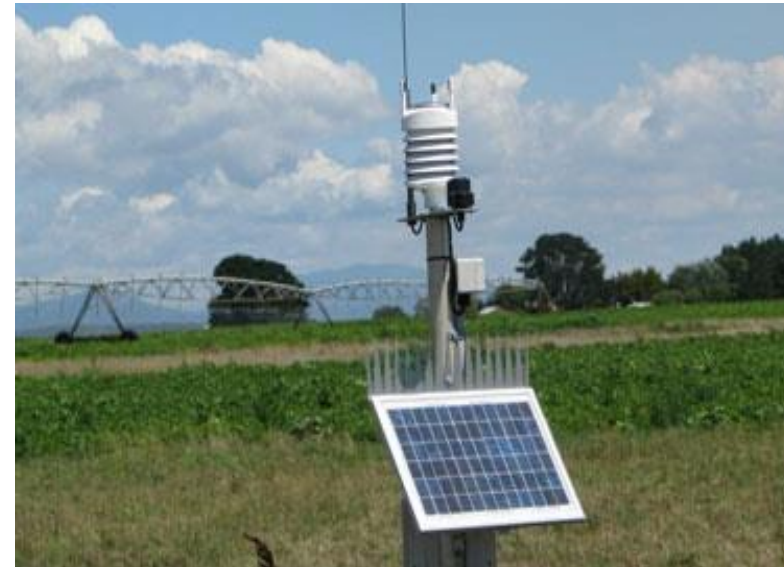
Installation example of Meteorological Station
